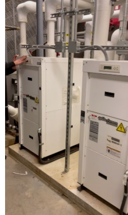
WATER SOURCE HEAT PUMPS
